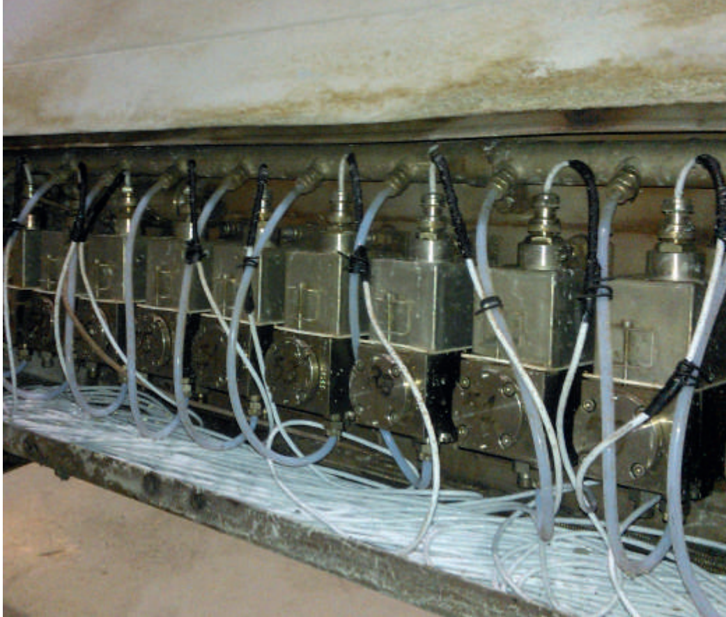
Figure 5. Original steam profiler actuators.
